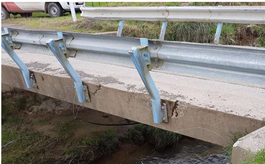
Figure 11-12 : Damaged side protection on Old Creamery Road bridge
