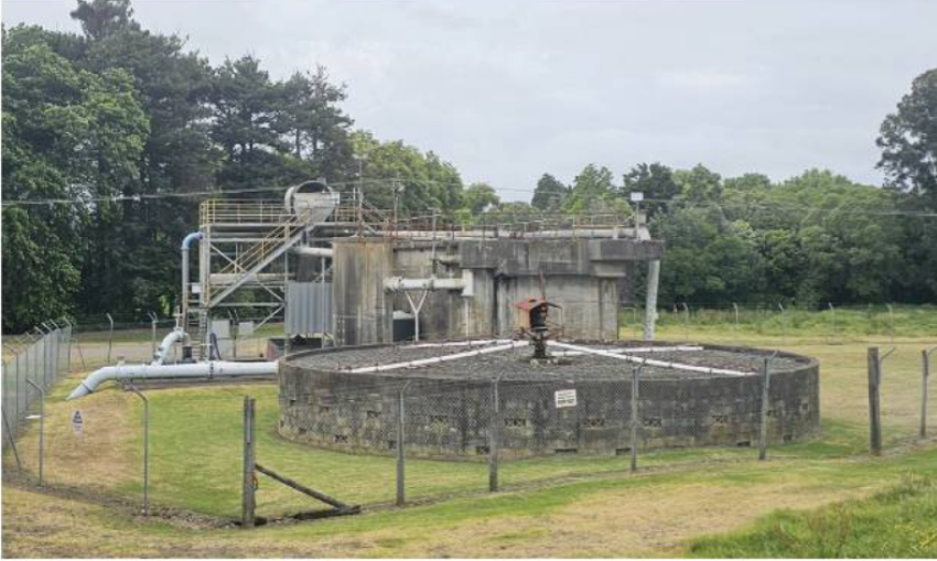
PRE-TREATMENT: Ōpōtiki District Council's wastewater treatment and pump at Whitikau Reserve will soon be receiving some upgrades.
